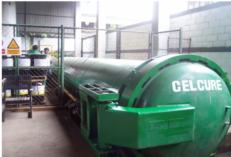
Plate 3.3: Vacuum pressure impregnation plant of Finlay Rentokil Ceylon (Pvt) Ltd
