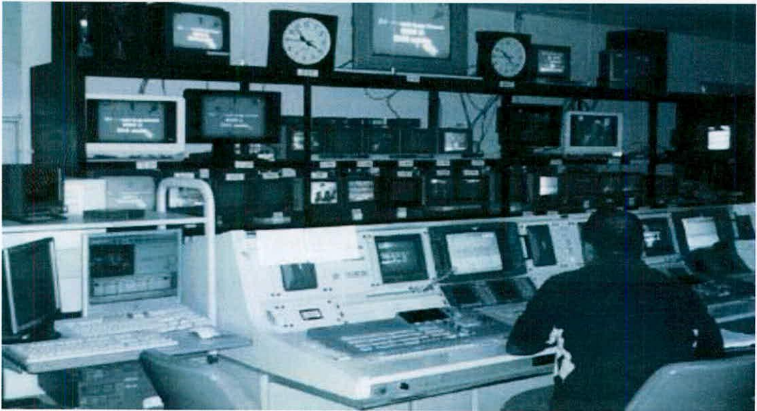
Figure 1 - Main Control Room
